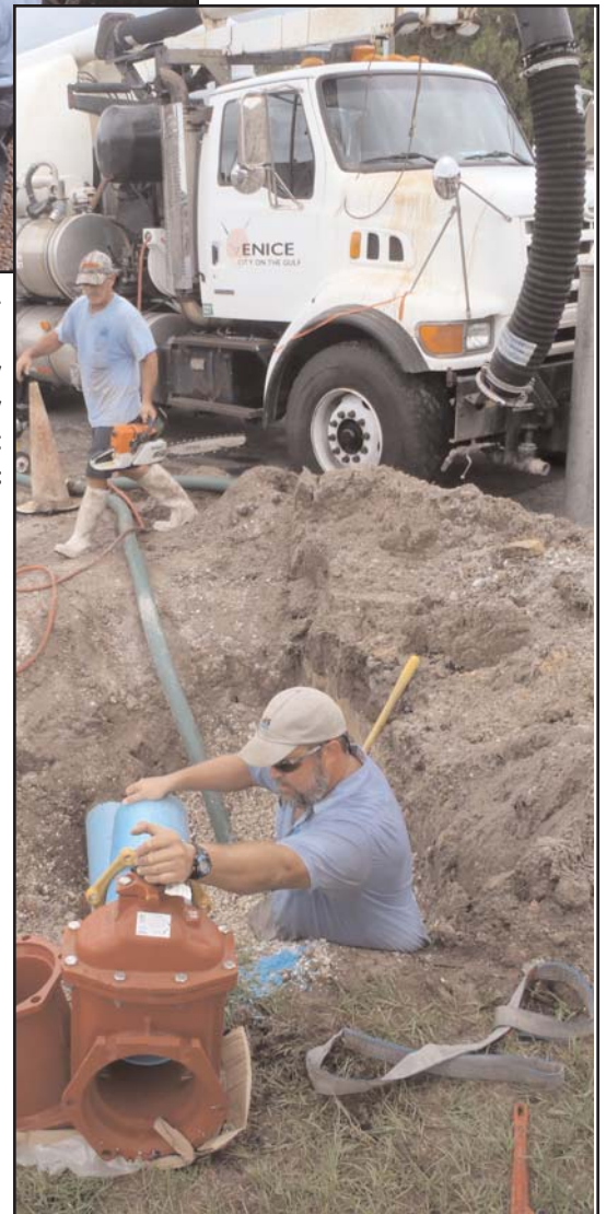
Eric Lindsay and Dave Guilmette prepare to install an eight inch gate valve into our water distribution system located at the reverse osmosis plant. This gate valve was installed to isolate the raw water pressure relief line from phase one of the water production plant.
