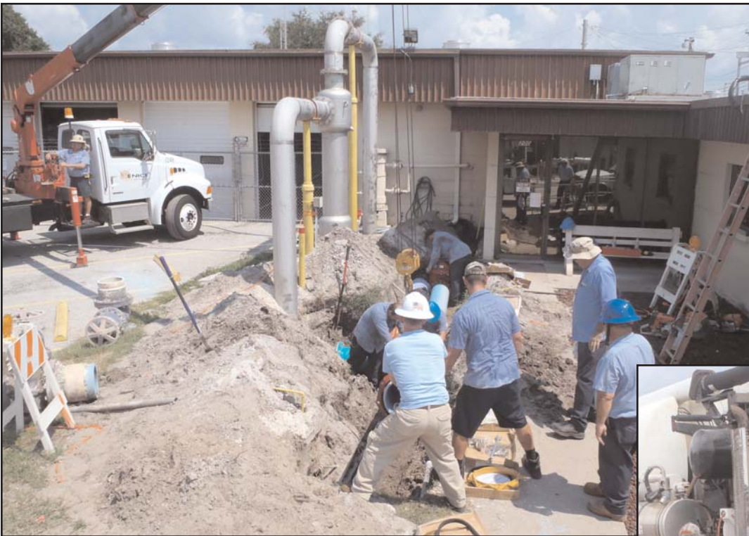
The Utility Department installs two 12-inch raw water valves that were inoperable due to excessive wear and usage. This is part of the valve exchange program that was a cost savings for the utilities department. From left, Bob Clark, Jeremy Petrosky, Ron Carter, Mike Sellers. In the work area are Phil Carnell, Tony Ramirez, Jimmy Bennett and Dave Guilmette. Wayne Hill operates the crane. Not pictured but a special thanks for their assistance and support, Brian Treat, Eric Barr, Gary Coble, Steve Park, Jim Anderson, Joe Stroer and Eric Lindsay.
