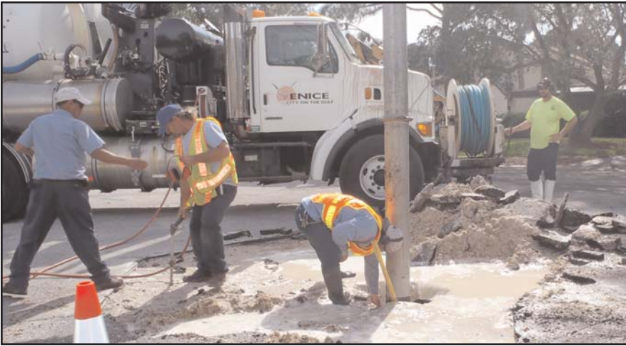
Field Operations team members repair a 1-inch service line in the 700 block of White Pine Tree Road. From left are Tony Ramirez, Marc Richard, Phil Carnell and Jeremy Petrosky operating the Vactor truck.
