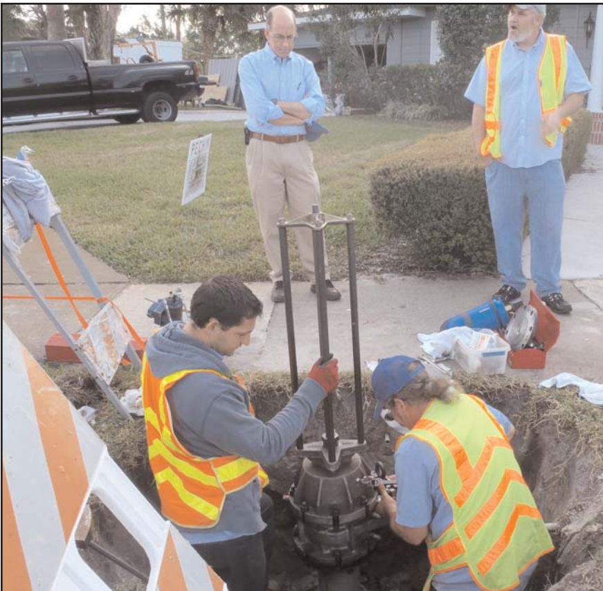
Vadim Bugayev and Marc Richard prepare to install a new 6-inch insta-valve in the water distribution system. This technology allows the installation without any disruptions to customers or the water distribution system. Assistant Utilities Director Tim Hochuli and Data Input Technician Damien Stillings are being briefed on the valve insertions process. The valve insertion took place at the corner of Harbor Drive South and Sorrento Street.
