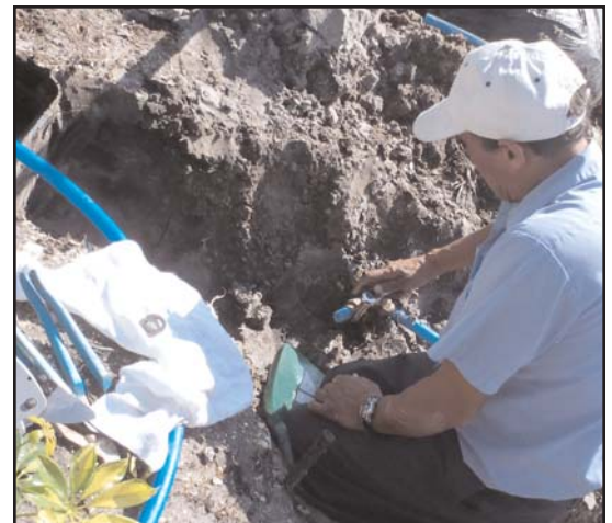
Tony Ramirez repairs a 1-inch water service line that a landscaping business accidentally damaged while planting a palm tree on Dante Street.
