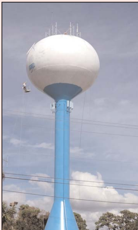
The city's 130-foot tall, 300,000 gallon water tank at the water production plant gets a new paint job.
